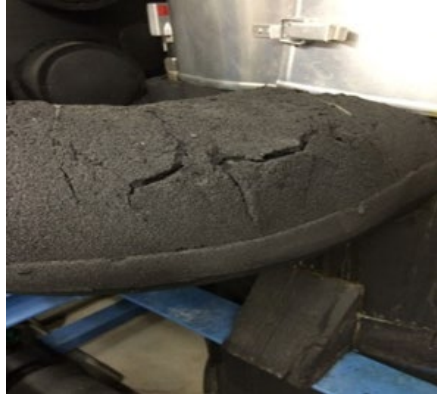
Condensation and corrosion
